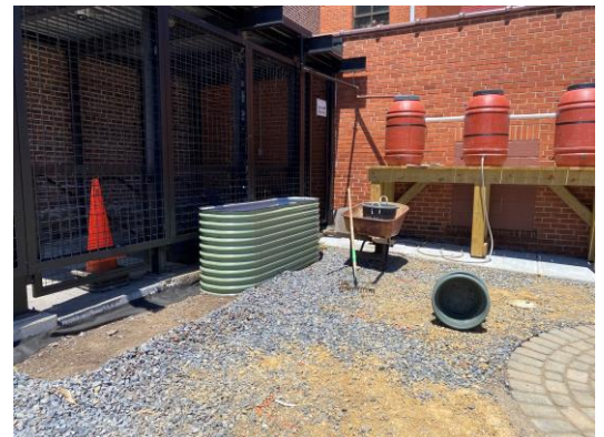
"During" picture with new rain barrel system, pavers, and raised metal beds for planting
